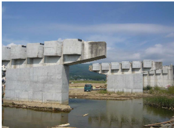
Figure 5. Damaged Numata-kosen bridge during Tohoku Tsunami
