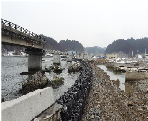
Figure 6. Utatsu bridge, the middle part was washed away
