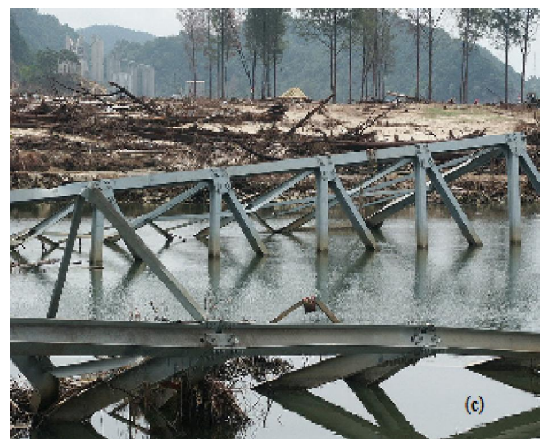
Figure 3. Bridge damage due to tsunami attack in Banda Aceh
