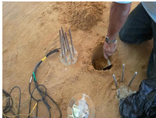
Fig (14) Placing load cell under cap Shuttering, reinforcement and concrete for Piled-raft cap directly in contact with soil Group (2).
