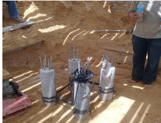
Fig (13) Placing piles and keeping the distance between piles (3diameters from enter to center) for Piled-raft cap directly in contact with soil Group (2).
