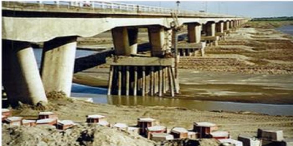
Fig (2) Effect of erosion and scour.
